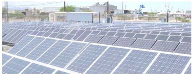
Figure 1. The TEP solar test yard. Over 600 PV modules from 20 different manufacturers are grid-tied, for a combined 90 kW peak . The yard, located at 4350 E. Irvington Rd, Tucson, AZ 95702, was commissioned in 2003. Photo credit: Alex Cronin, NREL PIX 17433.
